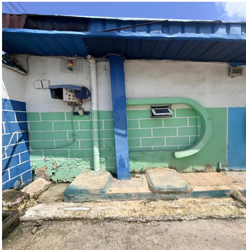
Plate 2.5: Drivers/loaders Facility Showing the Undersized Convenience Window
