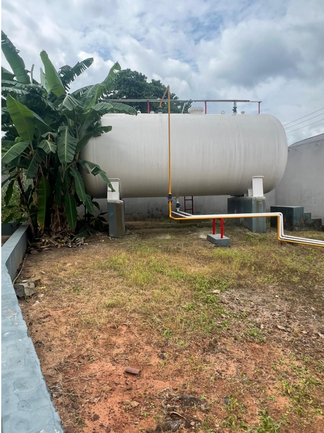
Figure 5. Storage tank with concrete stand support.
