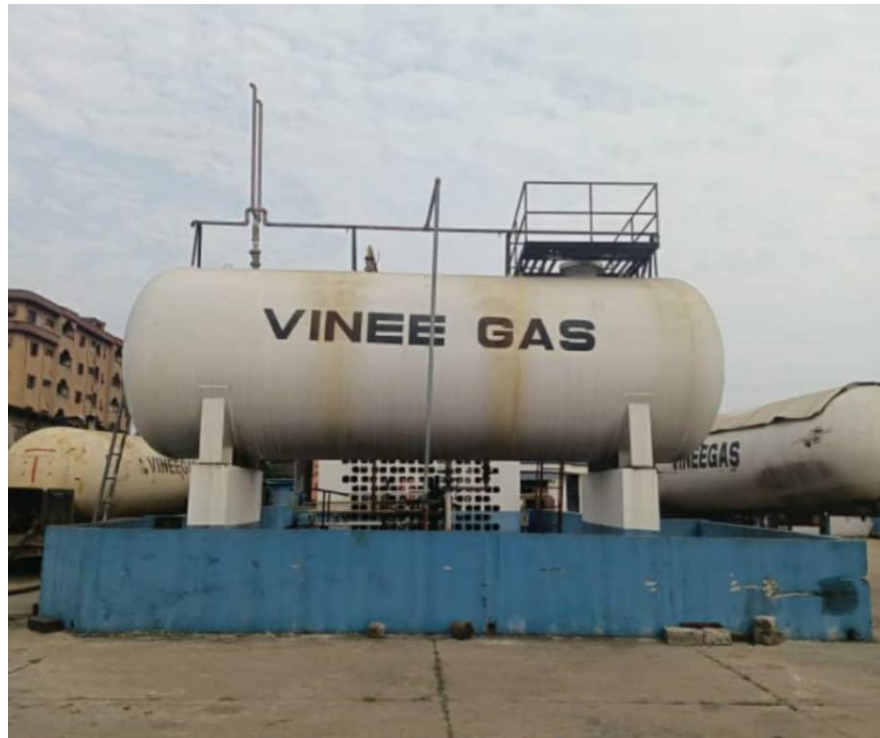
Figure 2.3: Storage tank at the Vinee Gas Plant Facility
