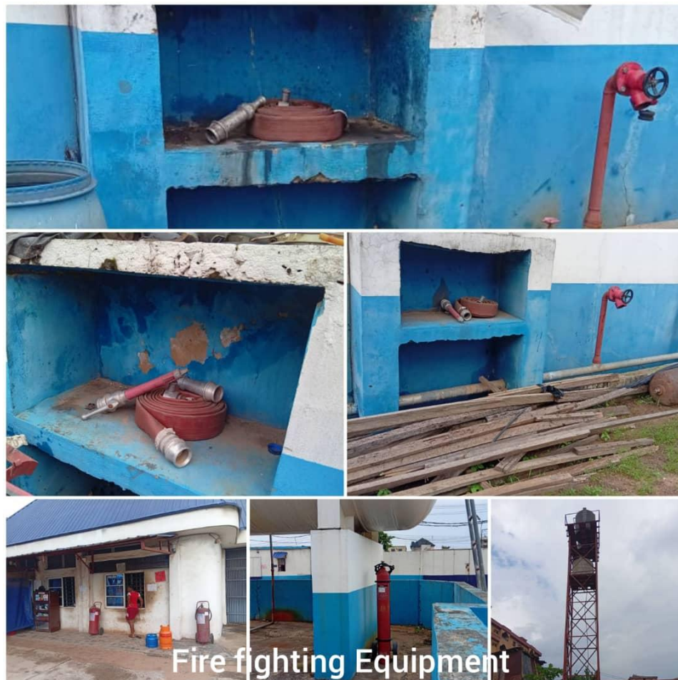
Figure 2.4: Fire fighting equipment
